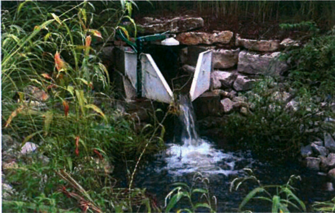
Stormwater BMP monitoring equipment at the Step-pool conveyance 2014.
