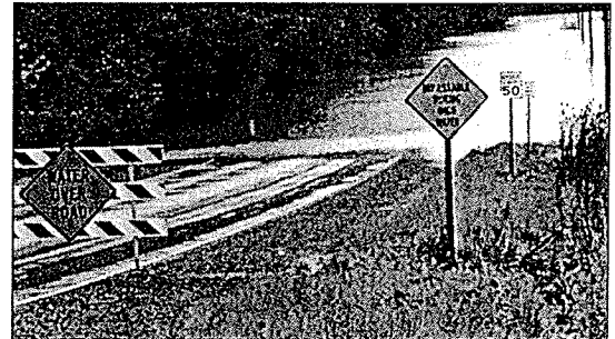
This photo taken from the Coats Lane intersection looking east is from 2014—one of many floods equaling or surpassing the "100-year flood" level.
