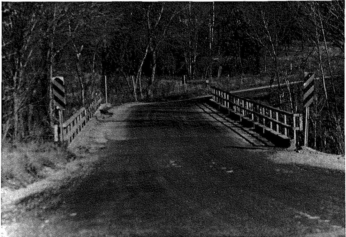
Photo 9 - This Boone County bridge is in acceptable condition but lacks pavement striping.
